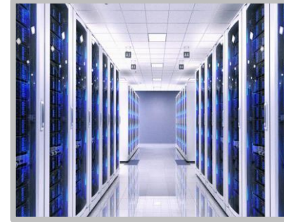
Data Centre / Cloud Hosting
